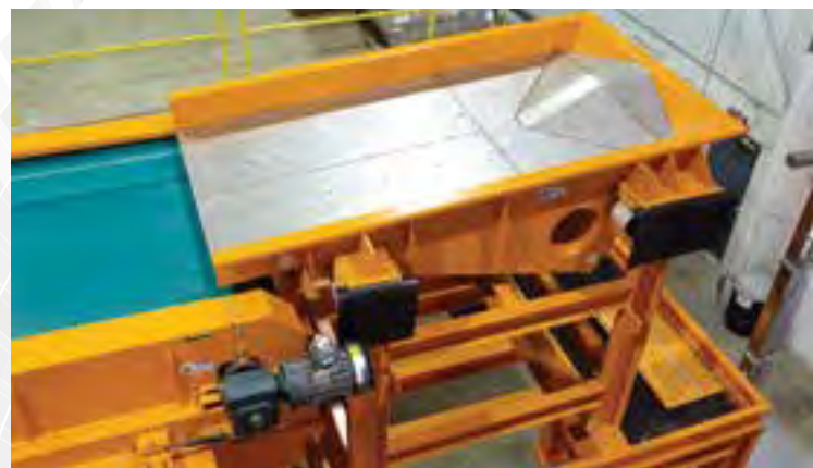
Diverters and liners can improve the spread of material and extend the life of the bed.
